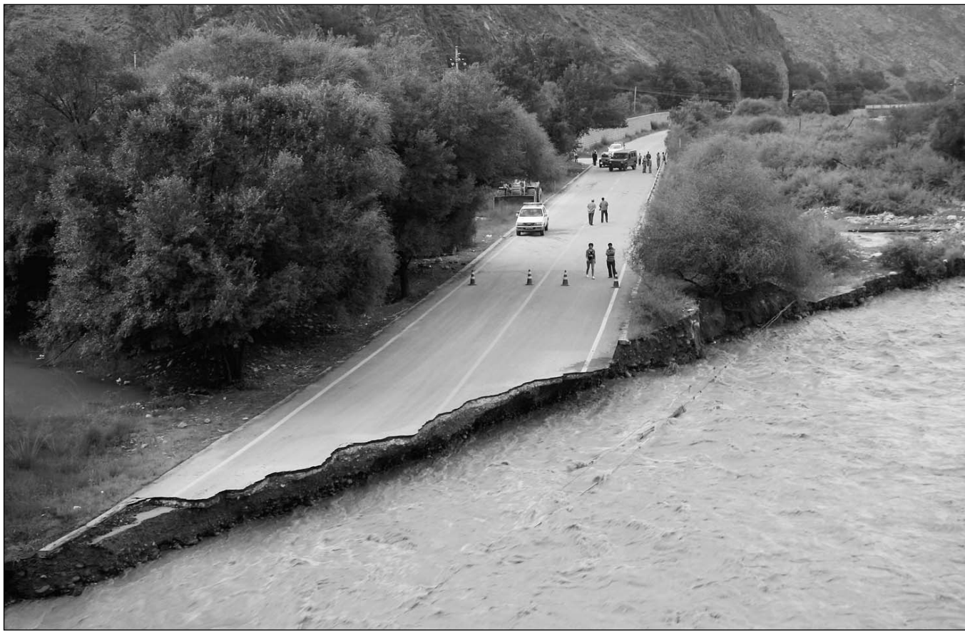
A section of the 218 National Highway, in Hejing county, the Xinjiang Uygur autonomous region, is severed by floods on early Saturday after continuous rainfall.
