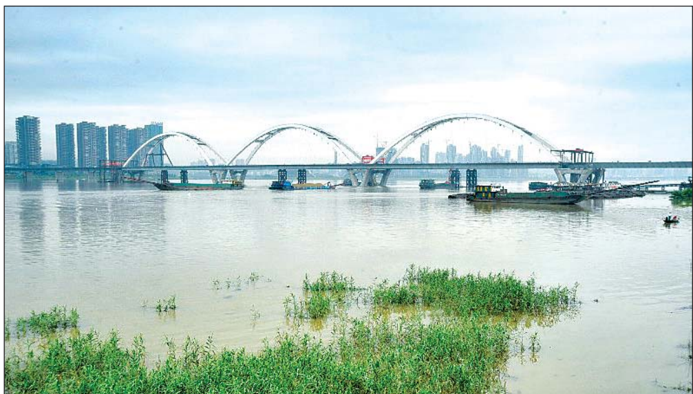
A bridge is under construction on the Xiangjiang River. When complete, the bridge will ease Changsha's traffic problems.
