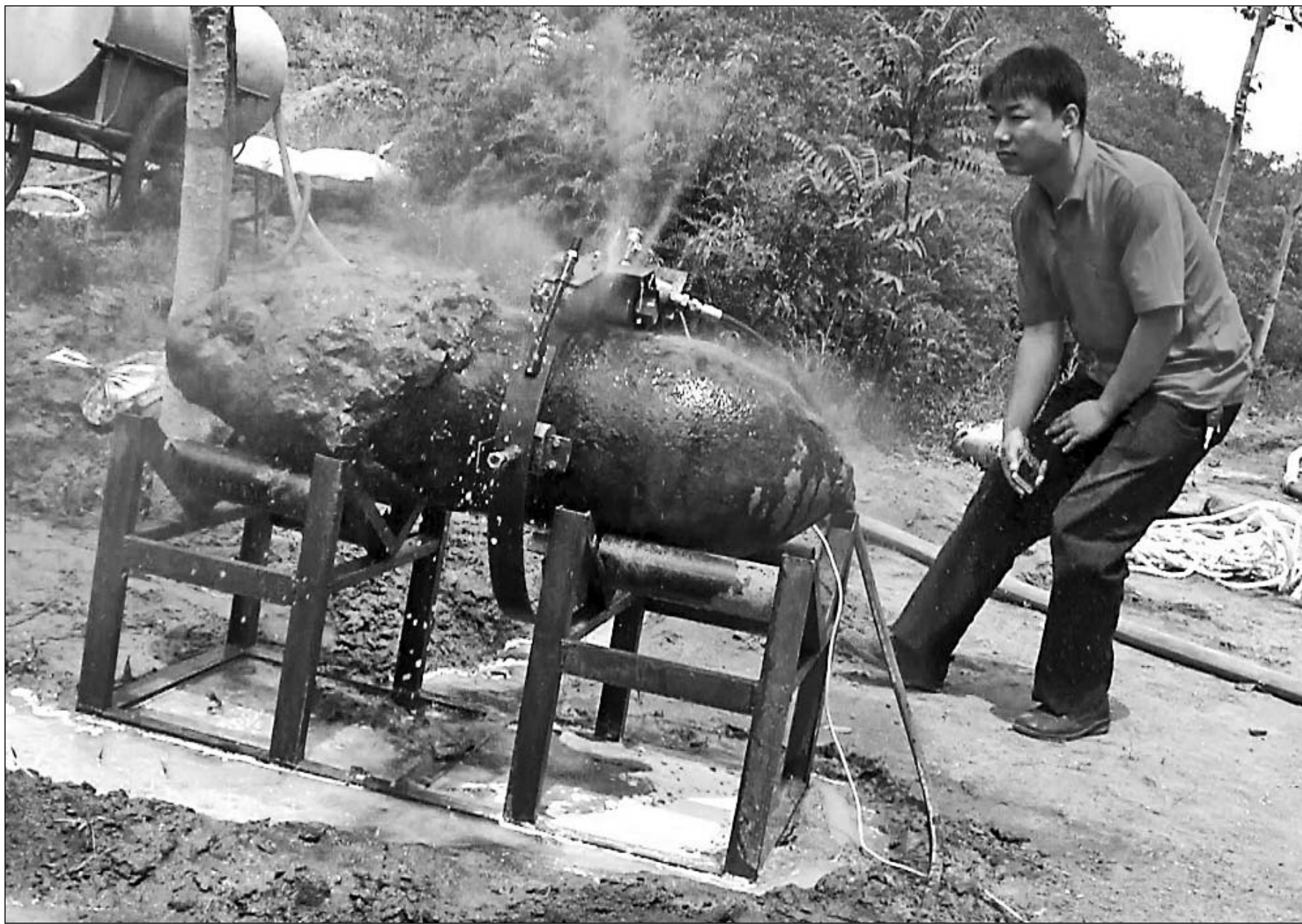
Ji Xingang uses his mobile water jet cutting machine to detonate a World War II bomb discovered at a construction site in Shijiazhuang, Hebei province.
