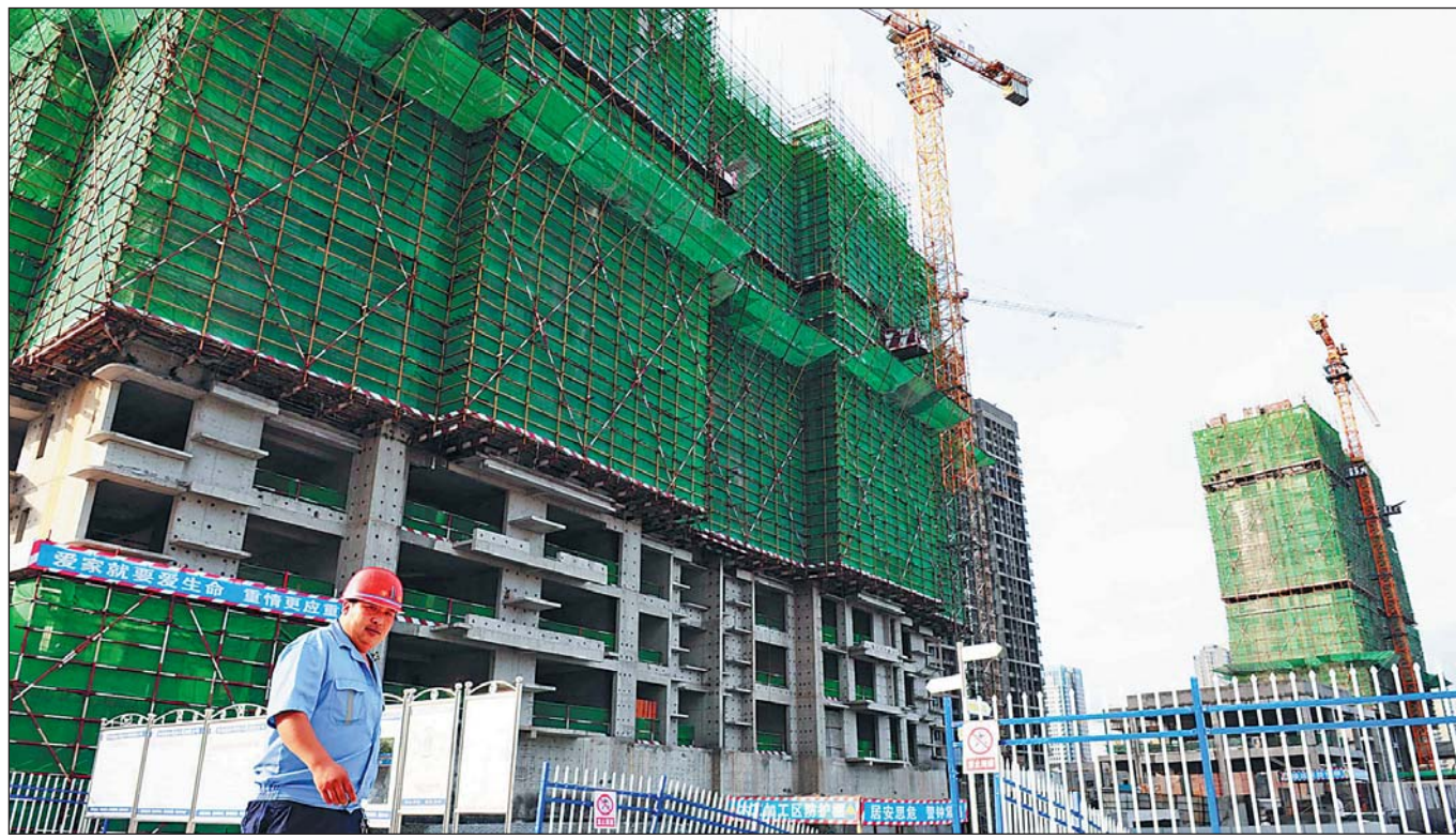
A construction worker at a housing project in Qingdao, Shandong province, on Wednesday. China's real estate investment grew 16.6 percent in the first six months of this year, compared with 32.9 percent growth in the same period last year.
